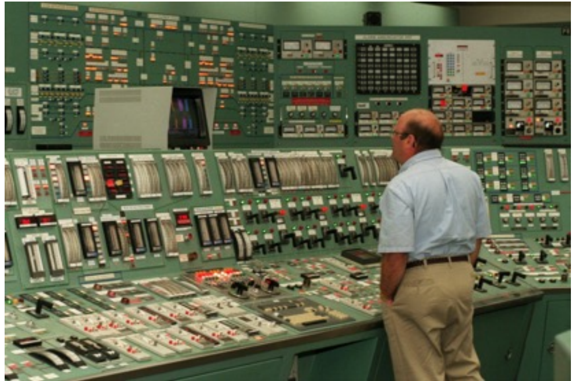
Three Mile Island control room.
